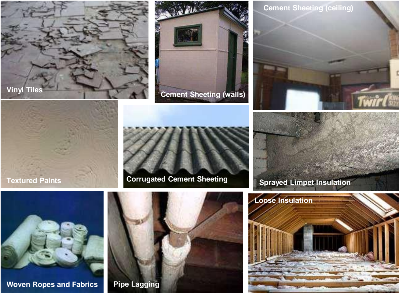
Figure 4 – Typical Asbestos Containing Materials (ACMs) from Bonded Vinyl Tiles to Friable Insulation
